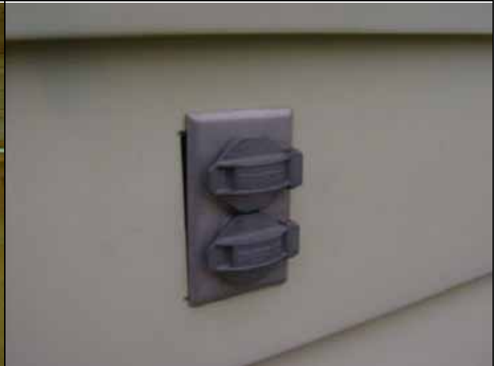
Loose outlet, needs GFCI protection
