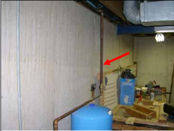
Pipes need additional support
