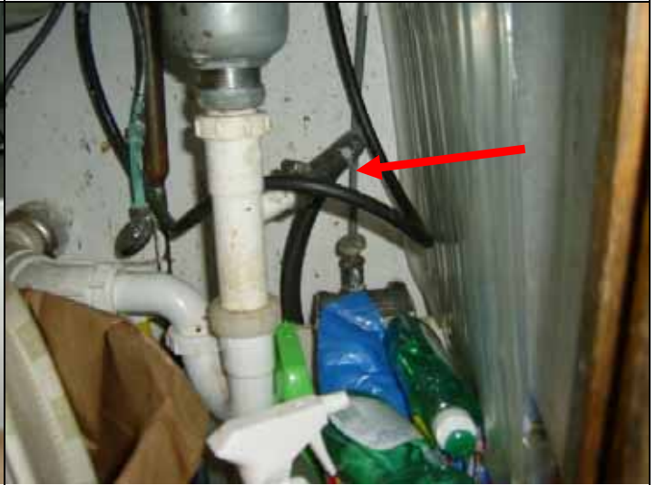
Improper dishwasher drain, add air-gap
