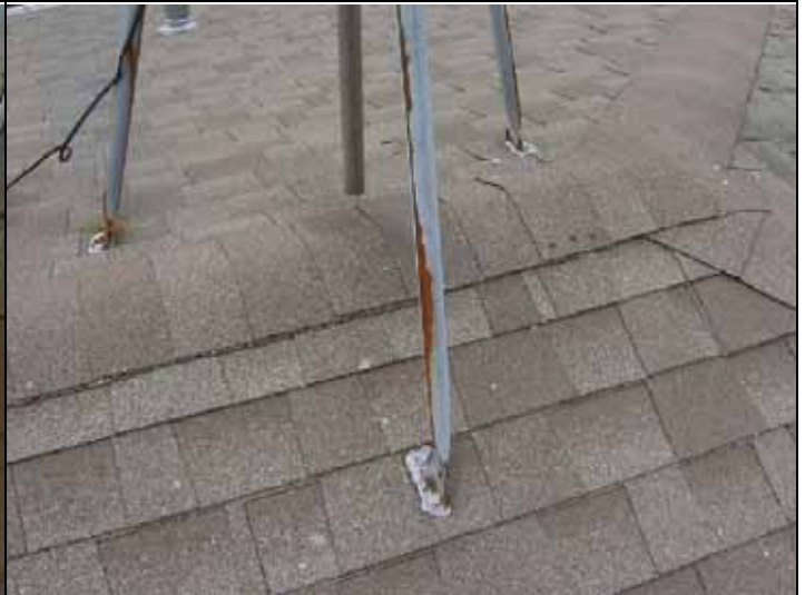
Antennae mounts need sealing
