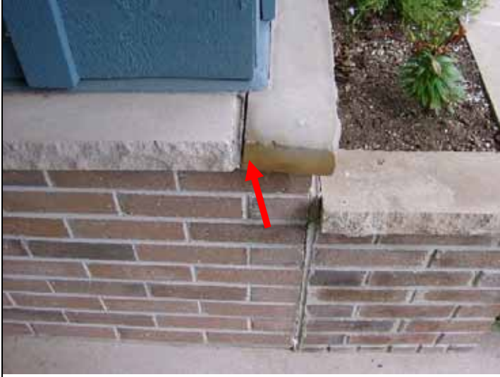
Some movement of joints
