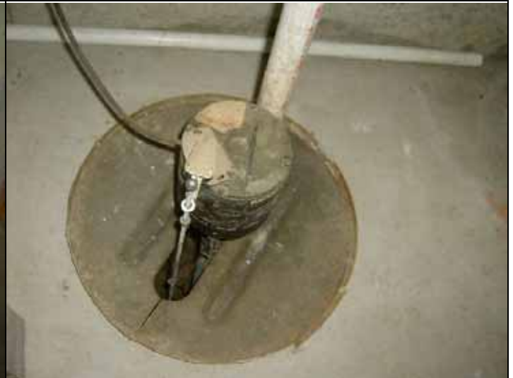
Sump pump failed
