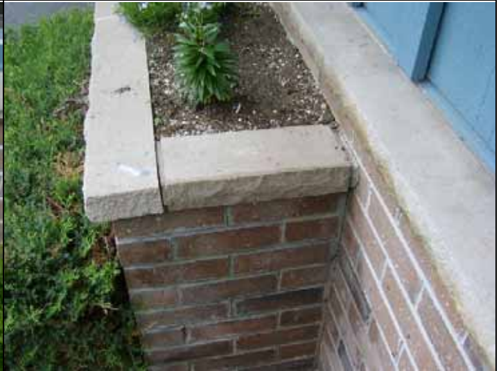
Some cracks, movement
