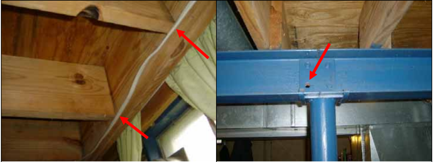
Add brackets, several similar locations noted Missing bolt
