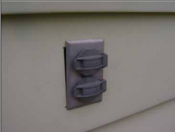
Loose outlet, needs GFCI protection
