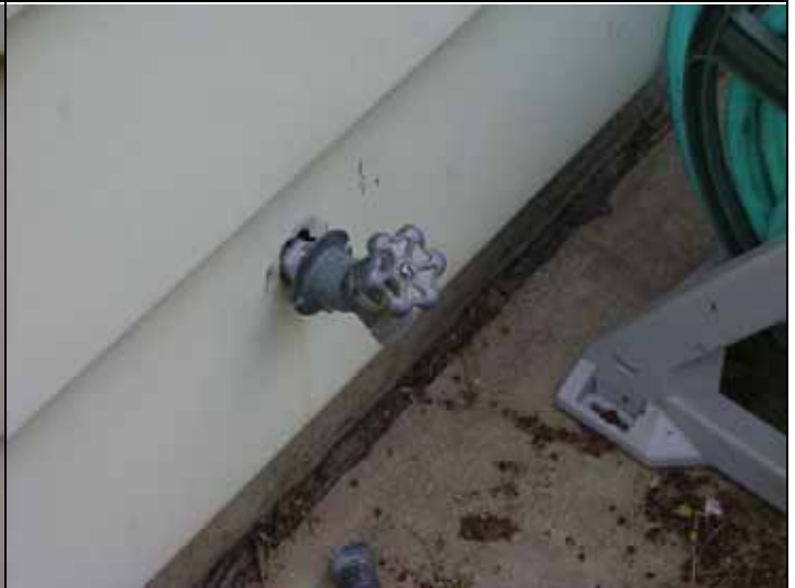
Caulk around pipe, needs vacuum breaker
