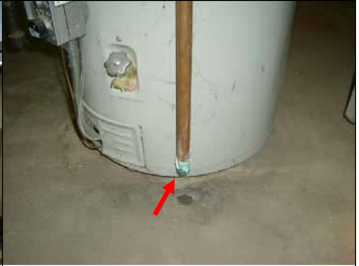
TPR valve leaks
