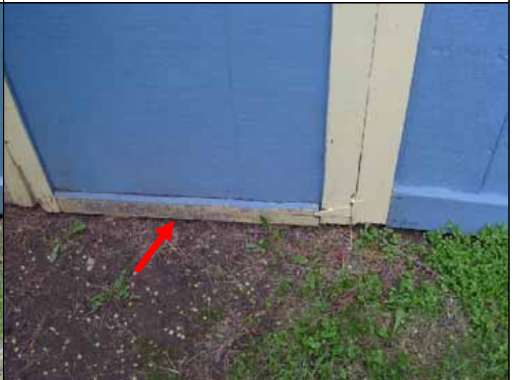
Wood rot on doors
