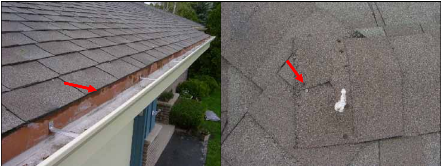
Rusted, reused flashings Exposed fasteners
