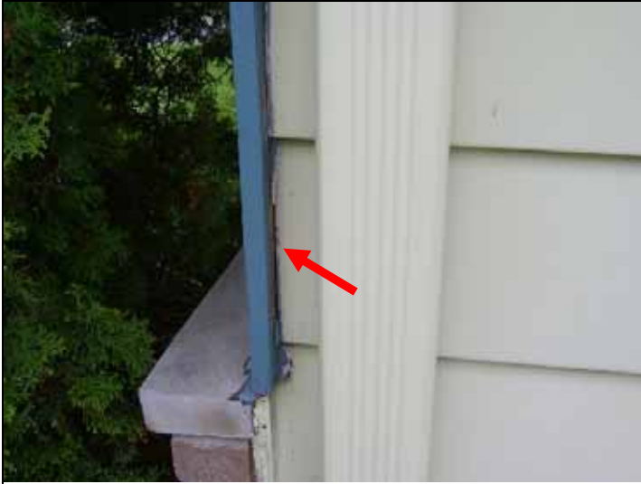
Gaps need caulk
