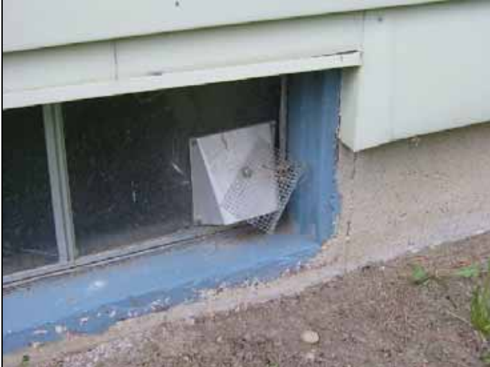
Replace dryer vent, needs damper and screen
