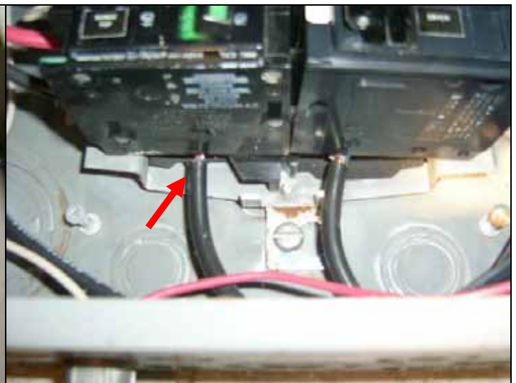
Sub panel wires improper connections and size.
