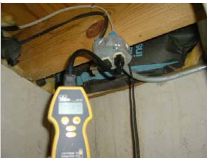
Sump pump and well pump had voltage drops of 14% other outlets had similar drops.
