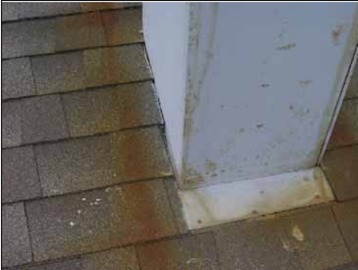
Chimney rusting, staining roof, pinhole rusted through on cap
