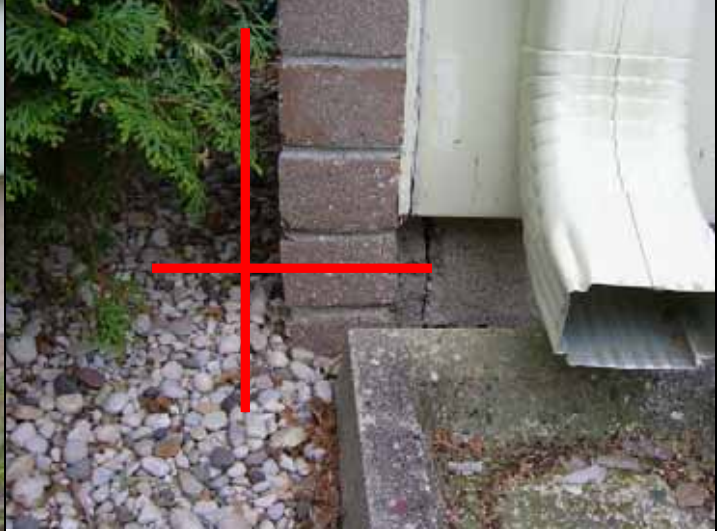
Minimal movement of brick veneer
