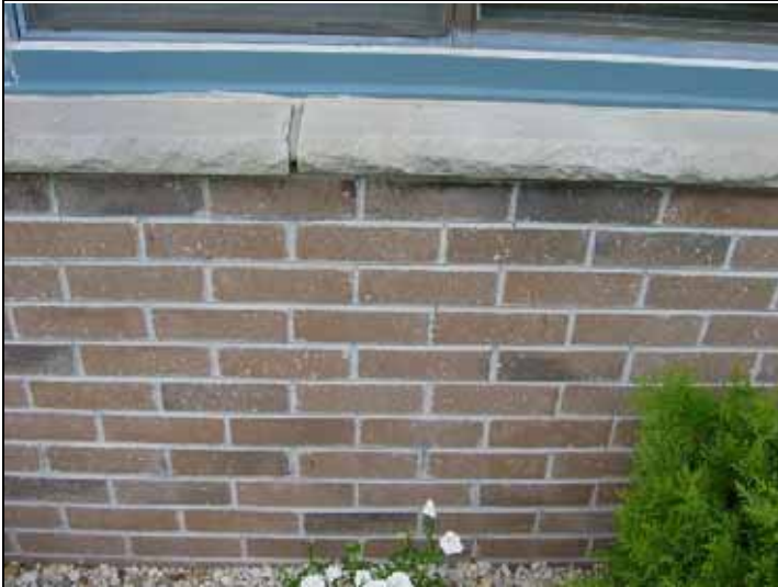
Deteriorated mortar joints, step cracks
