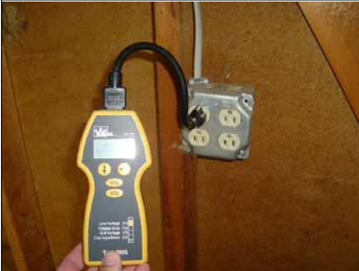
No grounds, loose, no GFCI
