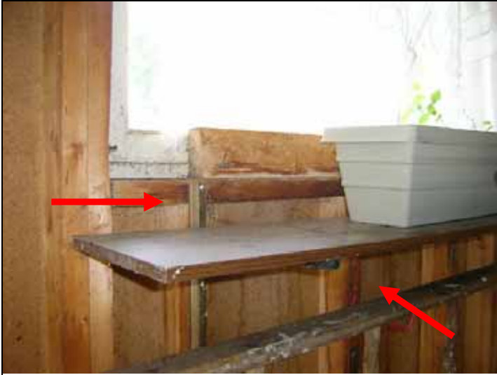
Signs of leakage around window
