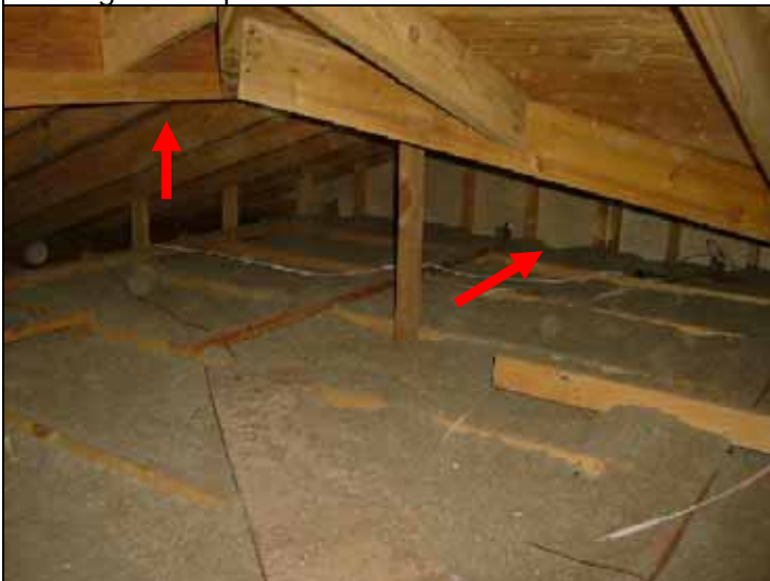
Garage wall as seen from attic, ridge board and valley framing support is improperly constructed
