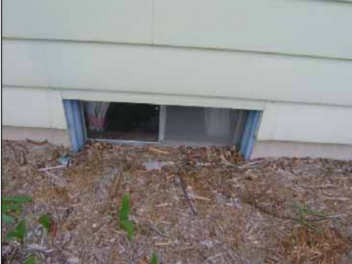
Clean and maintain around basement windows
