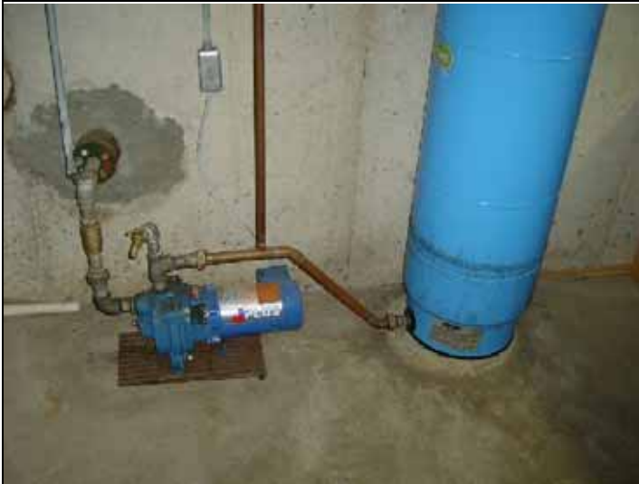
Shallow well pump and pressure tank
