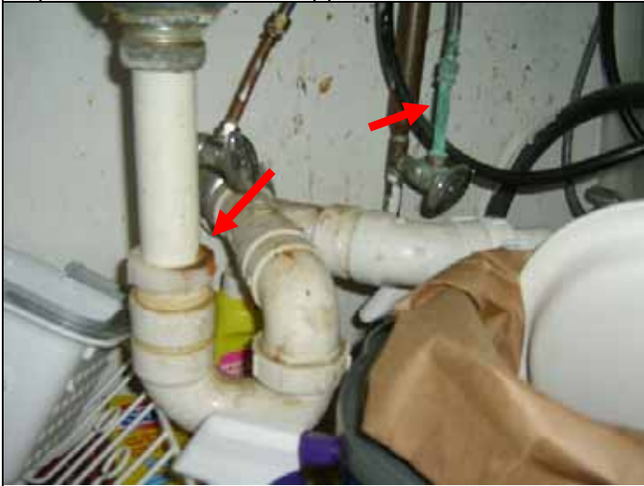
Corroded, signs of past leakage
