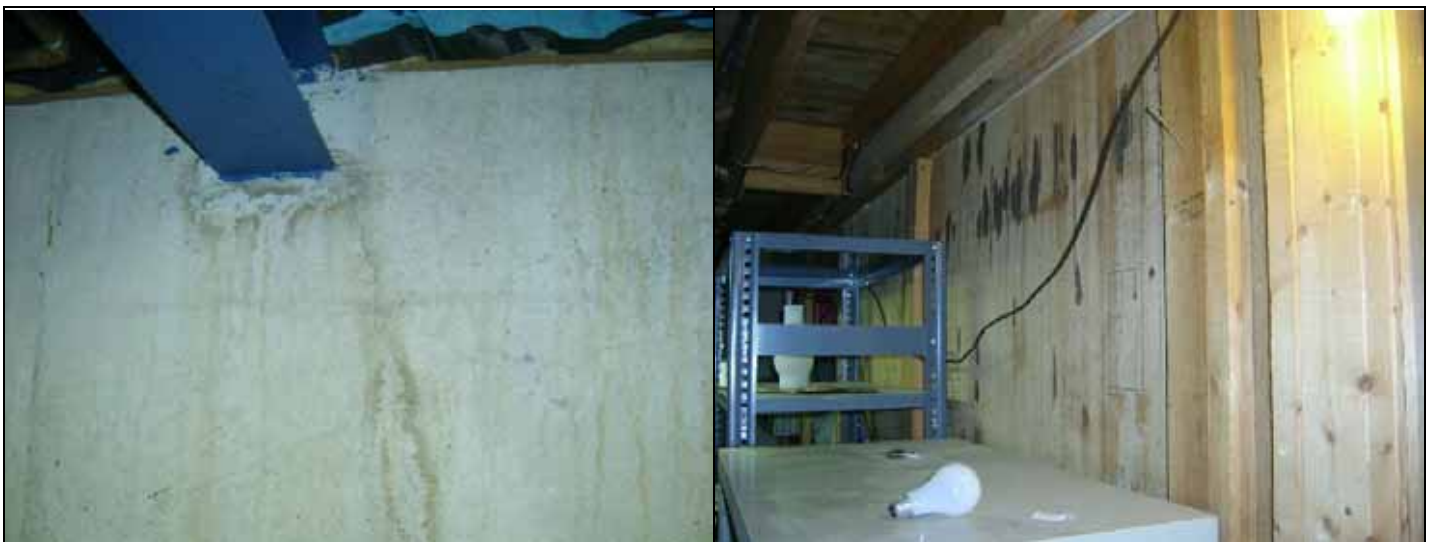
Some water stains on walls noted Partition wall lightly constructed
