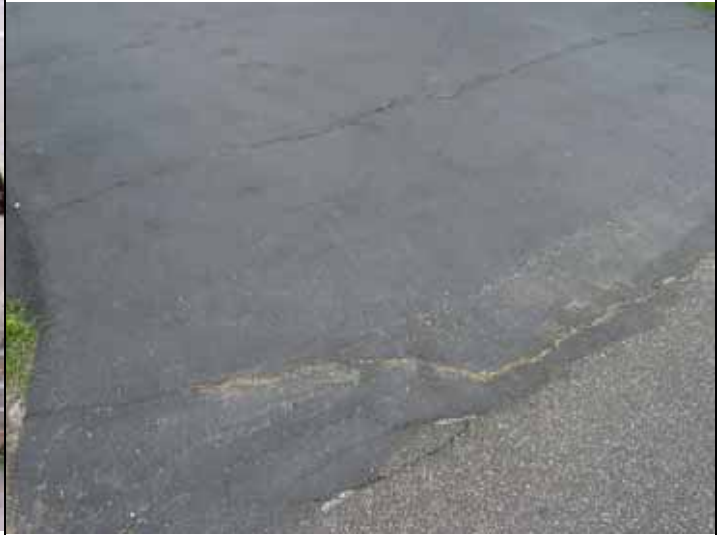
Driveway cracks and pitted
