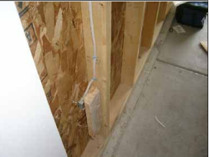
Exposed wiring in garage
