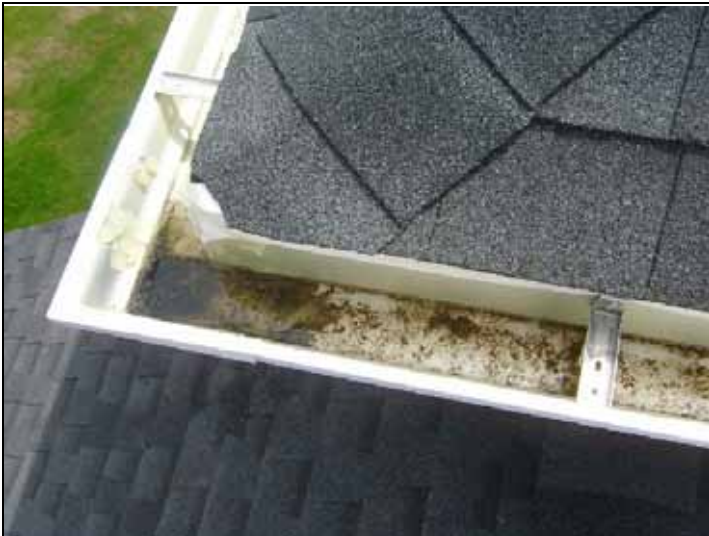
Improperly pitched gutter
