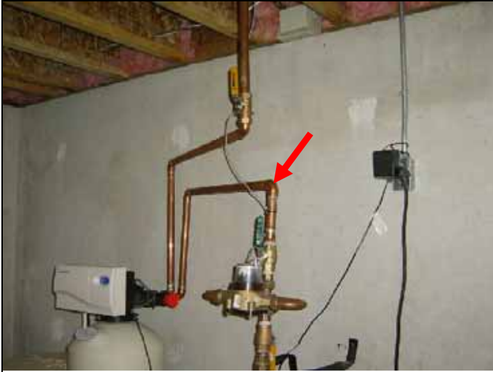
Water softener pipes need additional support
