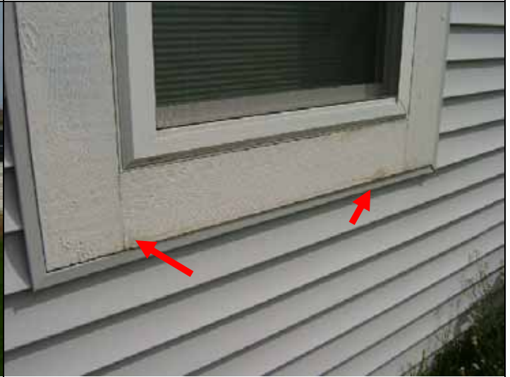
Discoloration on several wood trimmed windows.
