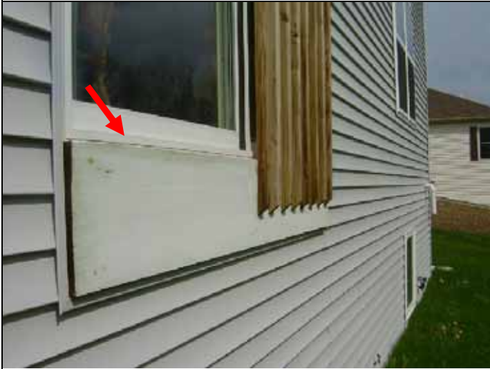
Deck ledger needs flashing and additional anchors
