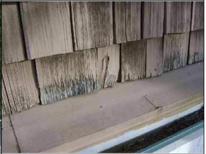
Deteriorated siding and loose metal flashing
