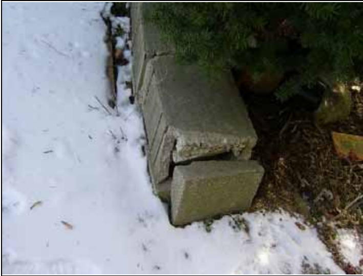
Retaining wall failed
