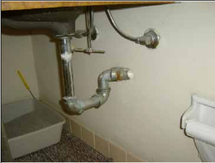
Improper drain, no shut offs
