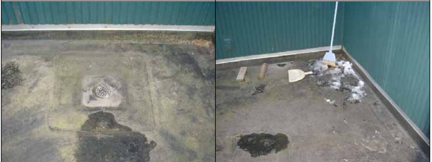
Keep drain clear Caution of ice build up and sharp objects.
