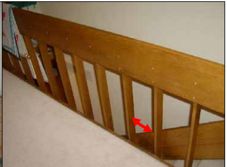
Balusters too wide
