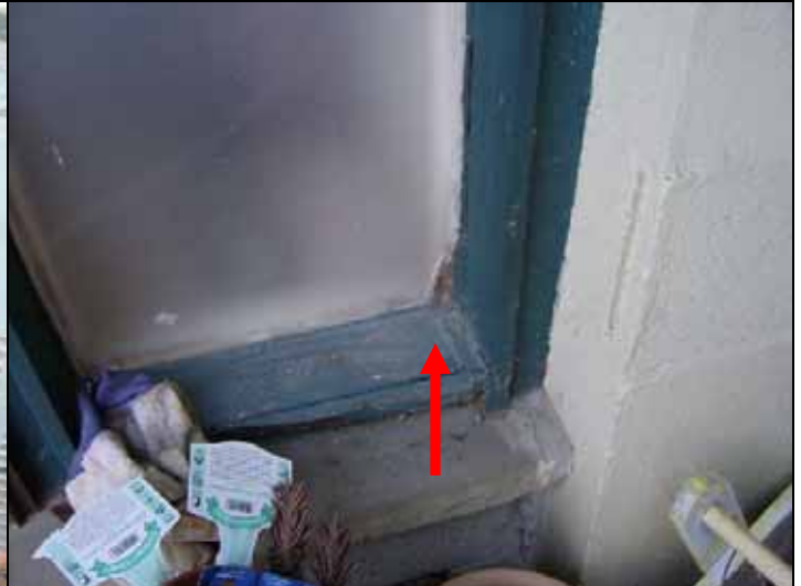
Sidelight window near rear door, wood damage
