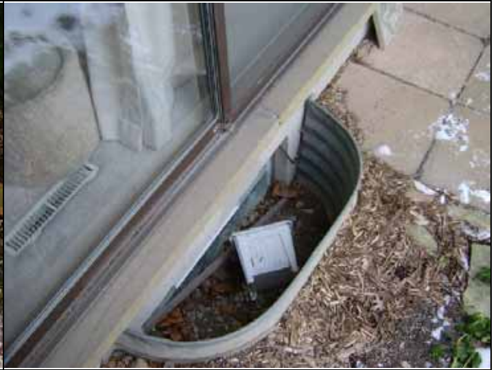
Window well low areas around patio and window well
