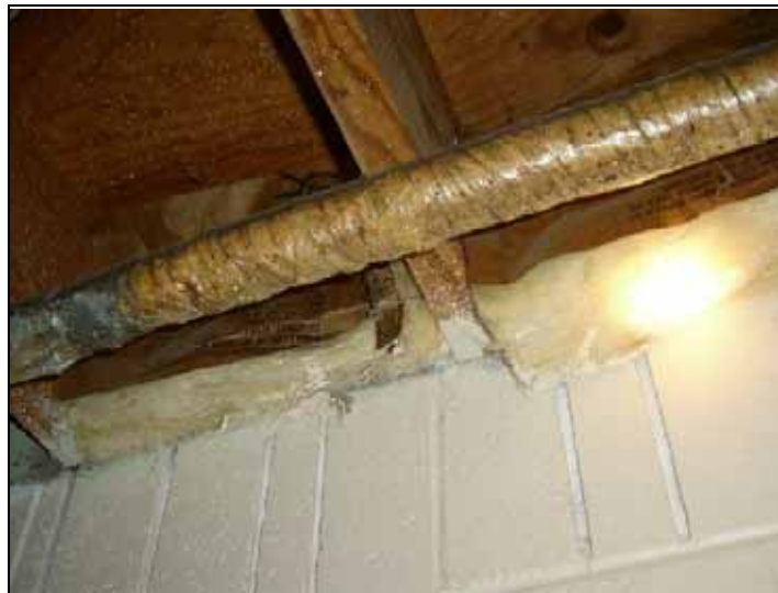
Fiberglass insulation and mold on pipe
