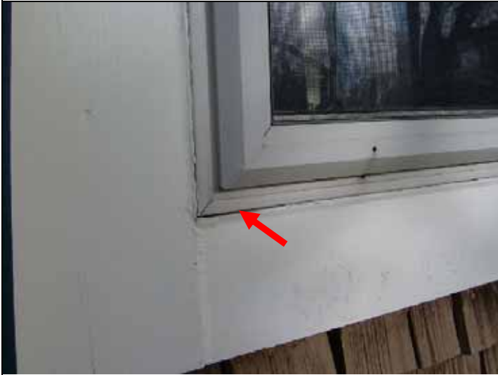
Minor caulking around windows
