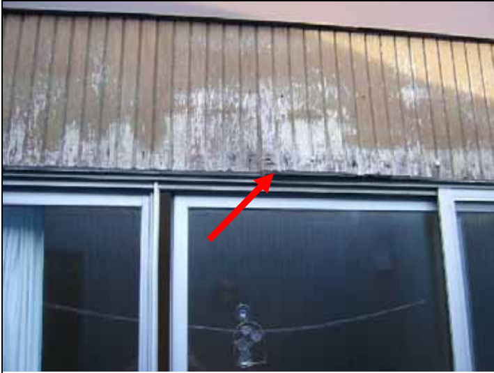
Deteriorated plywood above patio door
