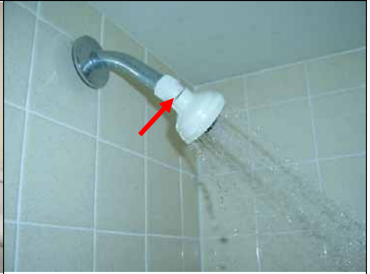
Leaking shower head.
