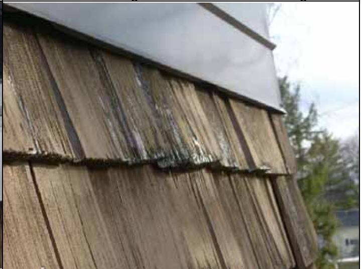
Deteriorated cedar shakes
