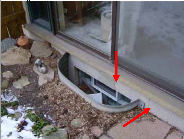
Missing step, trip hazard
