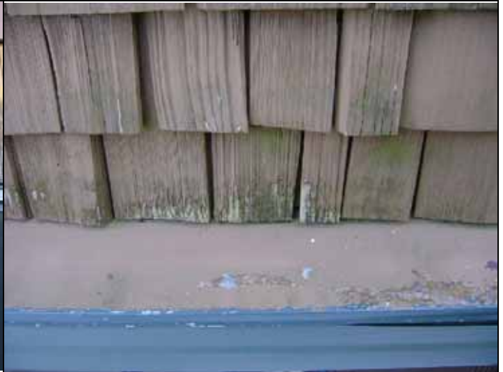
Deteriorated cedar shakes
