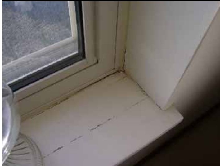
Sill damage in most rooms
