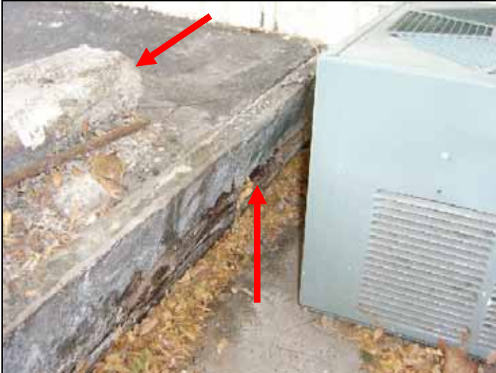
Parking area, deteriorated block and steel
