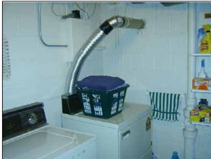
Dryer and venting, block panel
