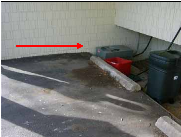
Parking area sloped toward the foundation
