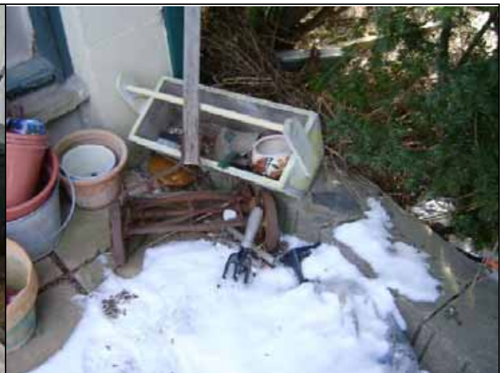
This area sunken and sloped toward the foundation.
