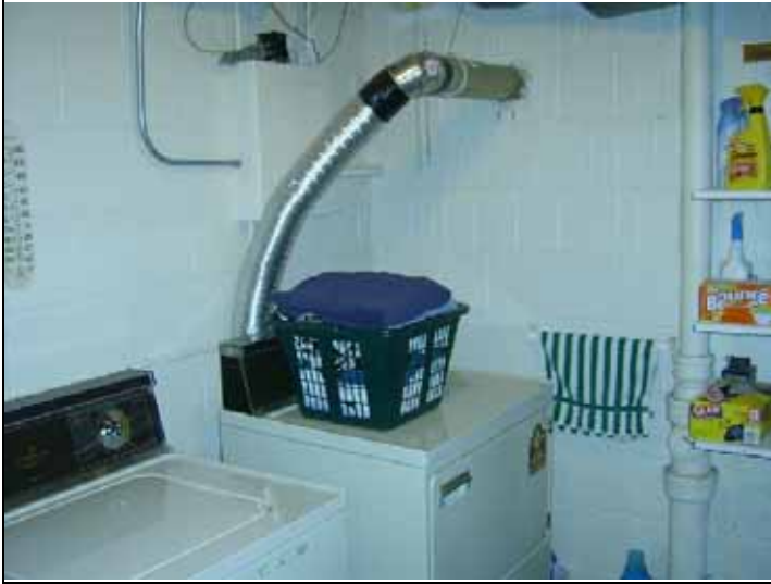
Dryer and vent obstructing panel
