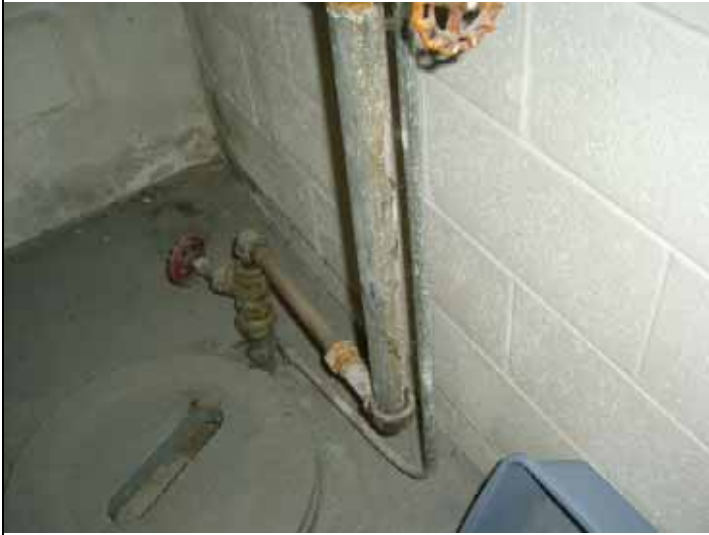
Southwest corner, sump crock, wall displaced
