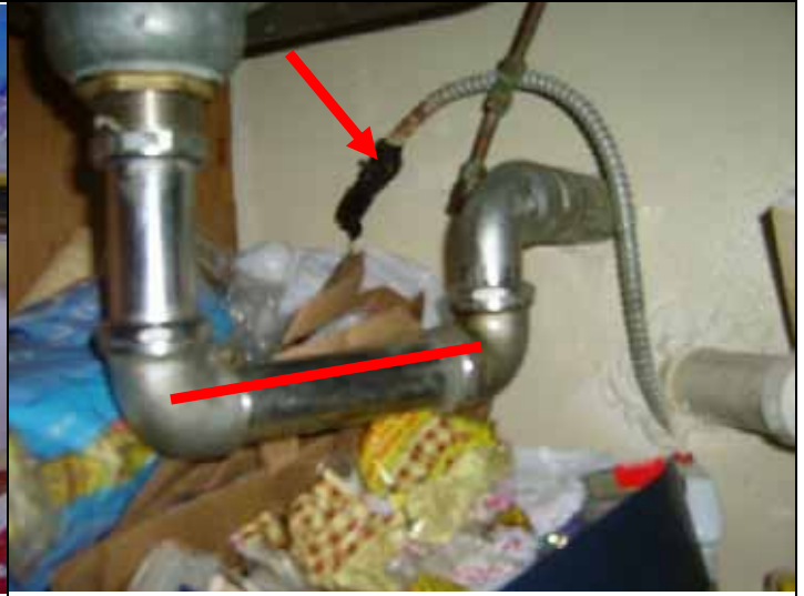
Improper trap, disposal wire
