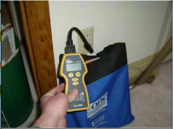
This outlet tested 10.9 % voltage drop.
