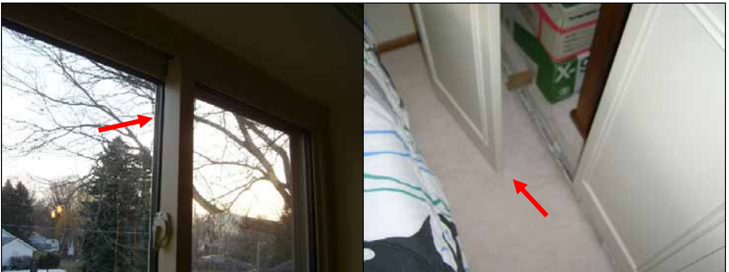
Windows not sealing, misaligned
