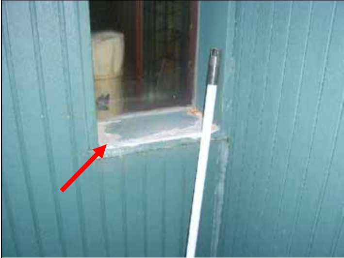
Deteriorated bathroom window
