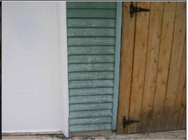
Fading siding, chalking paint
