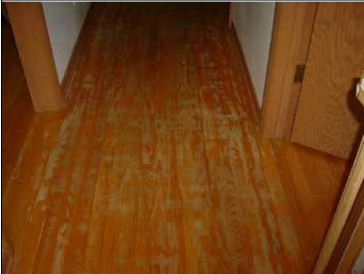
Deteriorated finish on wood floors
