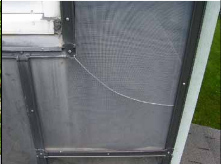
Several panes cracked
