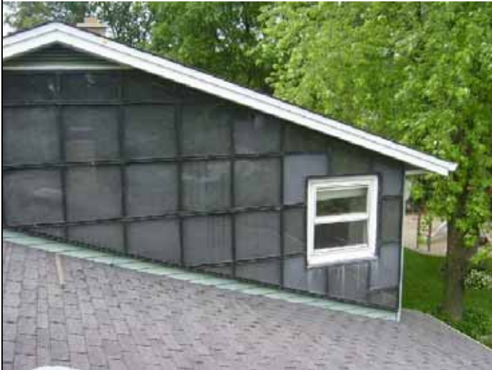
Solar heating panels damaged near window
