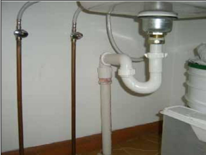
Hallway utility sink unvented
