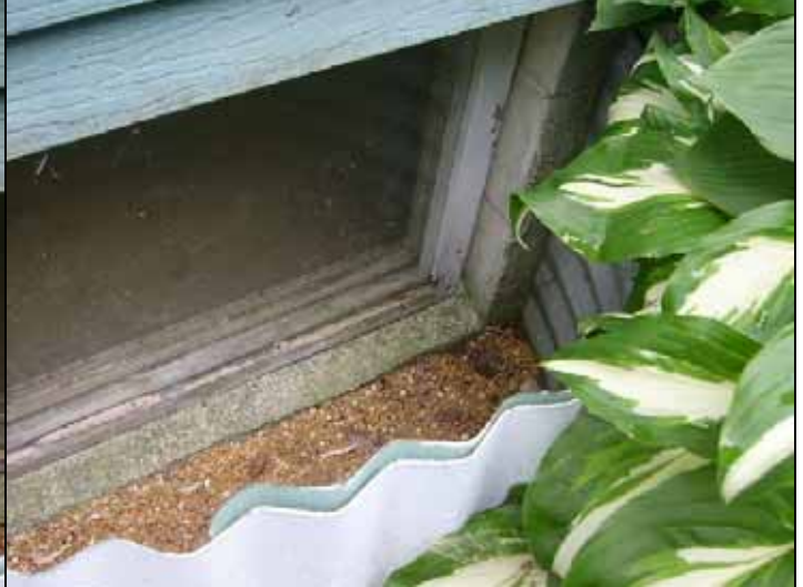
Wood rot evident in basement windows
