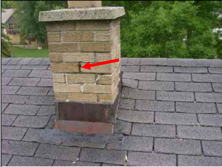
Chimney needs minor repairs and cap
