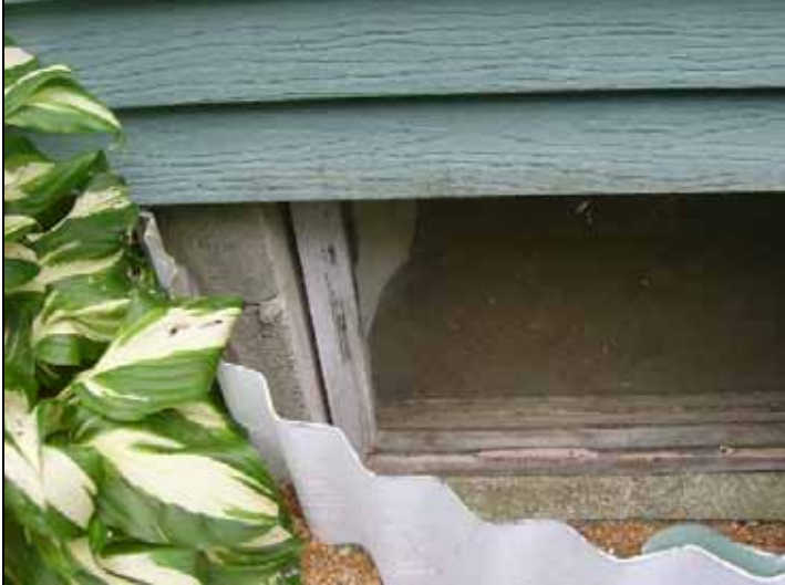
Basement windows deteriorated
