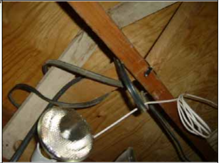
Flood light for crawlspace is fire hazard
