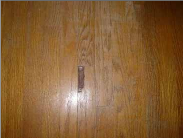
Minor defects in floor
