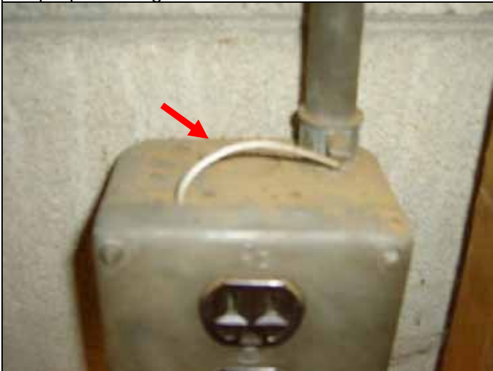
Small wire acting as ground
