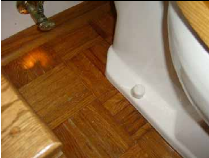
Water damage to floor
