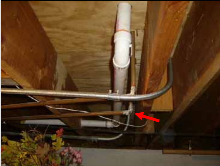
Improper drain, poor connections
