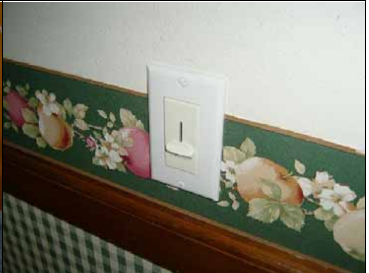
Dimmer feature not operational
