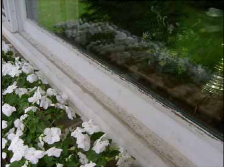
Large picture window sill, caulk and paint deteriorated.
