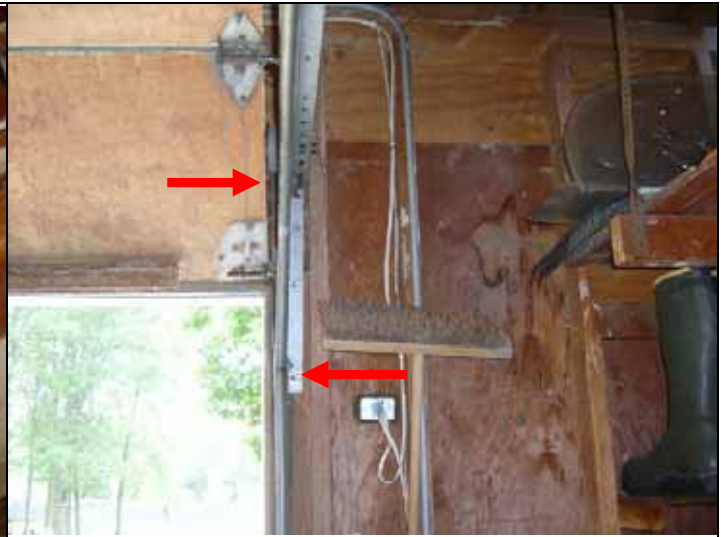
Garage track misaligned
