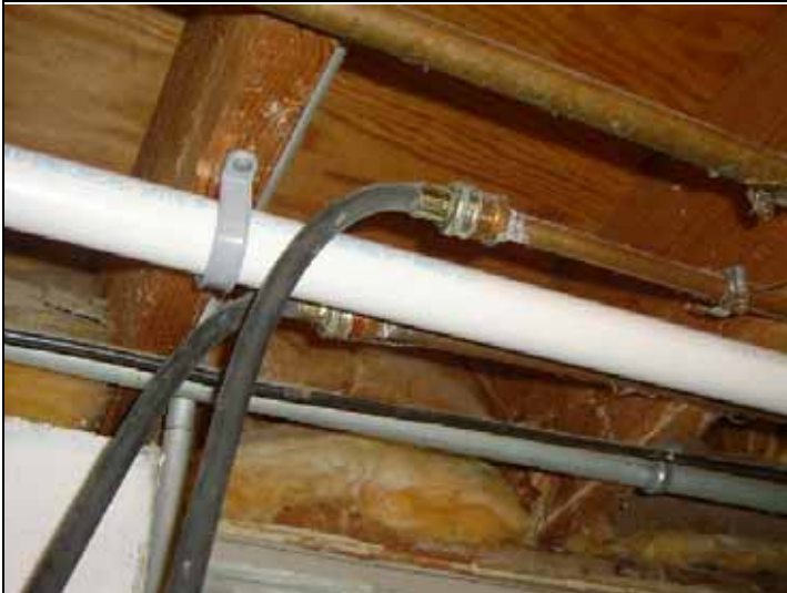
Hoses supply utility sink
