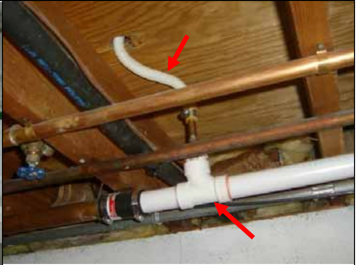
Improper dishwasher drain
