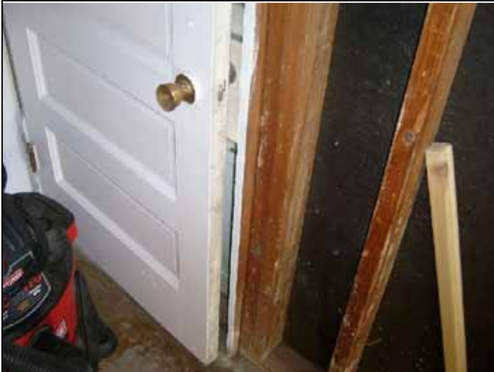
Door not aligned well needs adjustment
