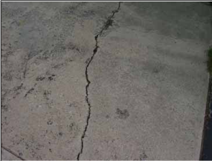
Cracks in concrete drive
