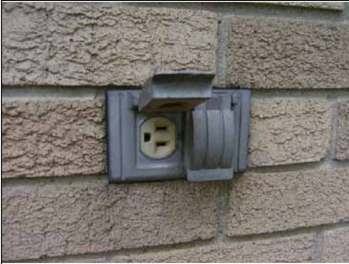
Ungrounded outlet, needs GFCI protection
