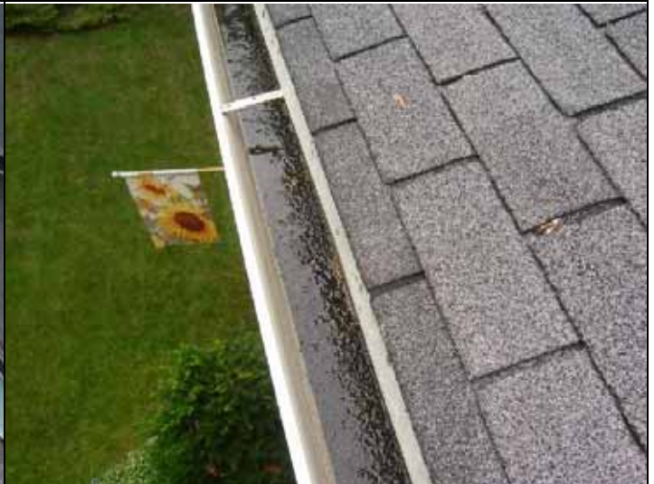
Gutters improper slope and granules
