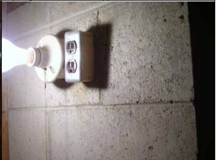
Cellar outlet, lighting, needs GFCI, damp location
