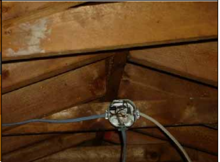
Open junction and unsupported wires in attic
