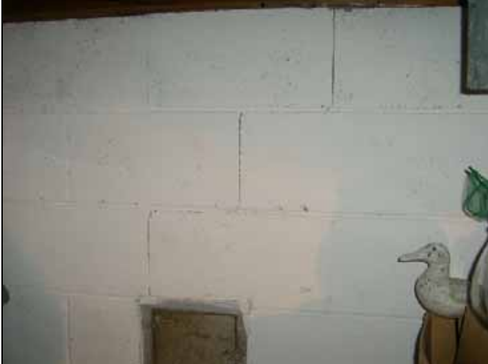
Step settlement cracks under chimney, fireplace
