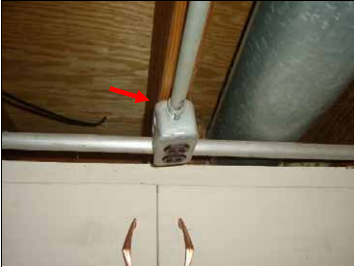
Loose outlet box
