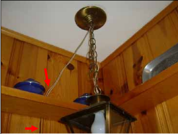
Improperly wired lamp
