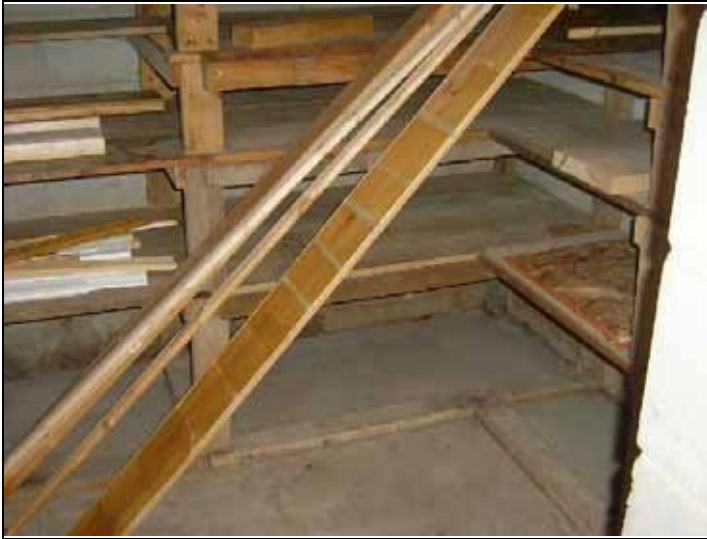
Untreated wood in contact with masonry
