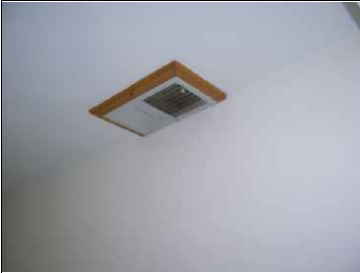
Solar air vent, possible moisture leakage
