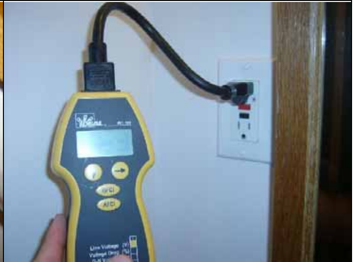
Failed to trip
