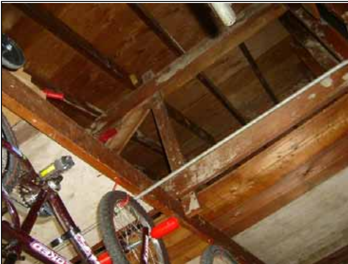
Storage area, inadequate framing
