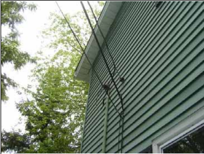
Service drop appears to be 60 amp
