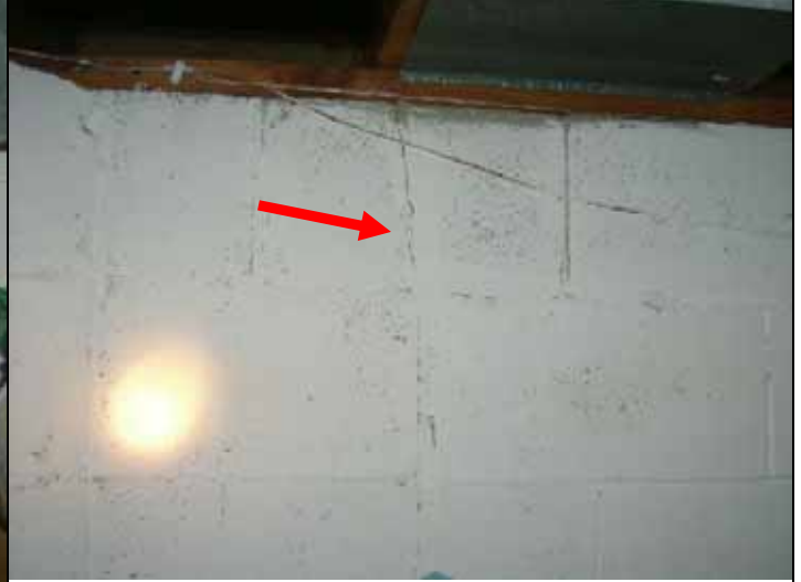
Old crack repair
