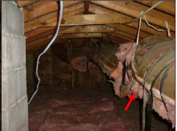
Solar ducting in attic
