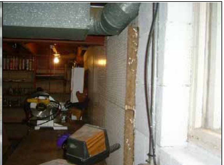
Bowing visible in peg board area
