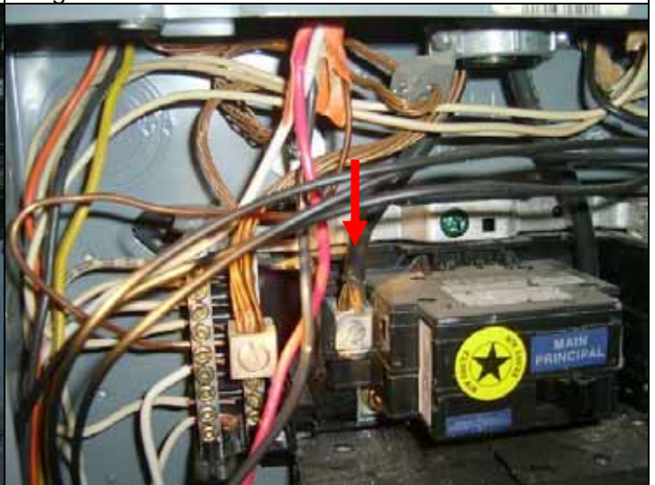
Poor connection, sloppy wiring
