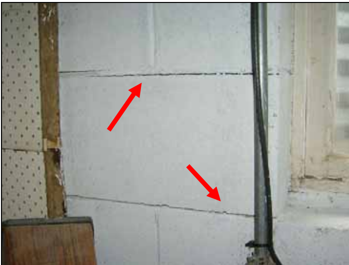
Horizontal cracks in wall
