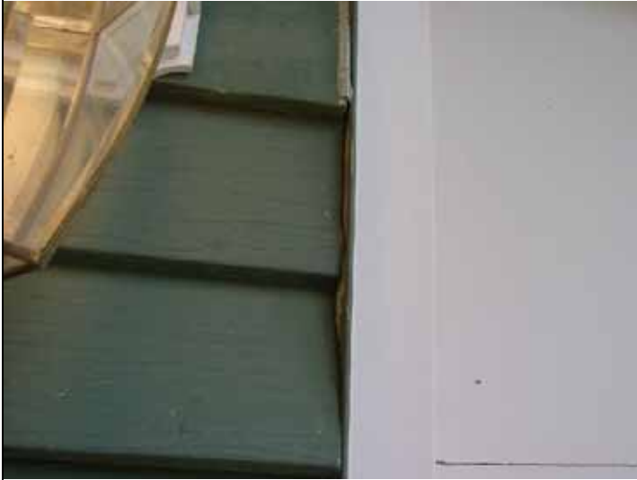
Example of caulking needed
