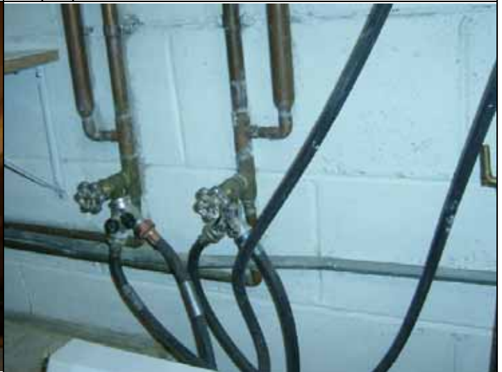
Washer and utility sink supply
