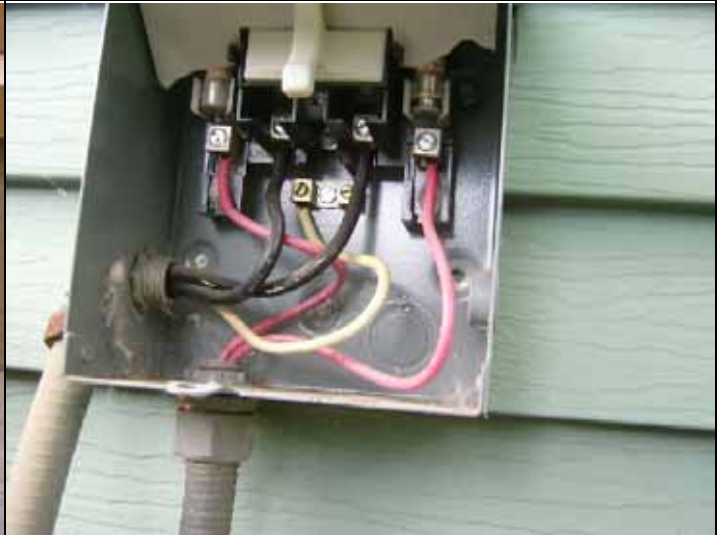
Ungrounded AC disconnect
