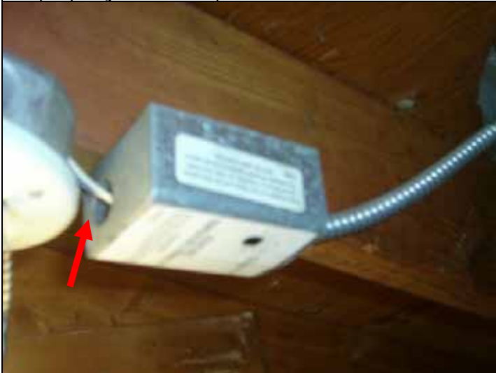
Improper wiring to attic fan thermostat
