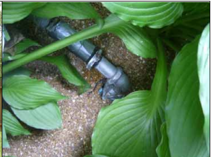
Sump discharge line
