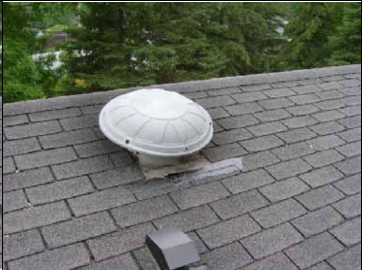
Power vent hood
