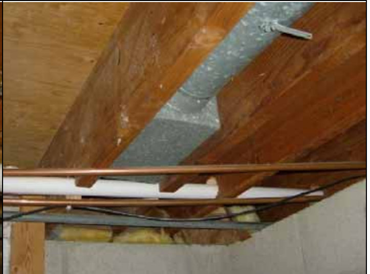
Improper drain and joist notching weakens joist
