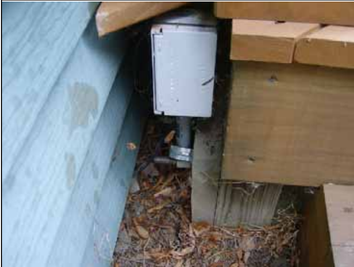
GFCI outlet not operational
