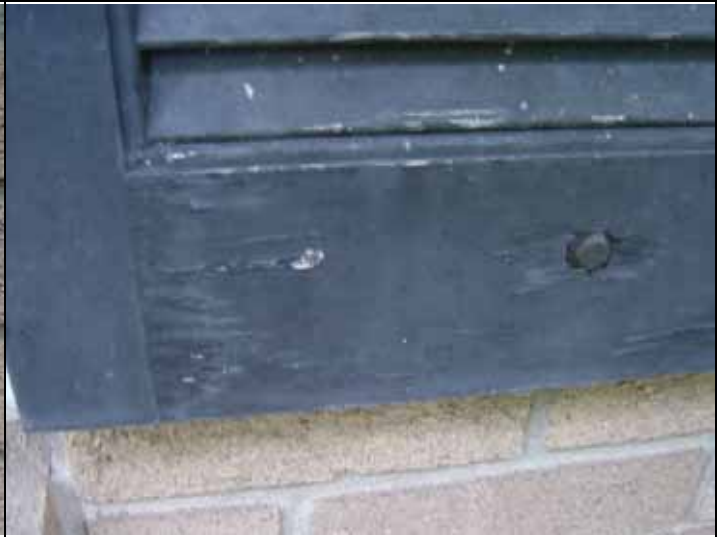
Example of shutter condition
