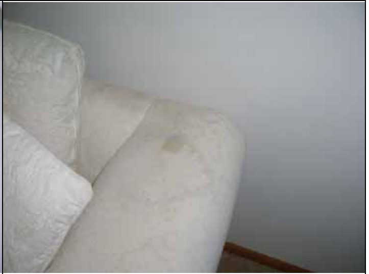
Drips on couch beneath vent
